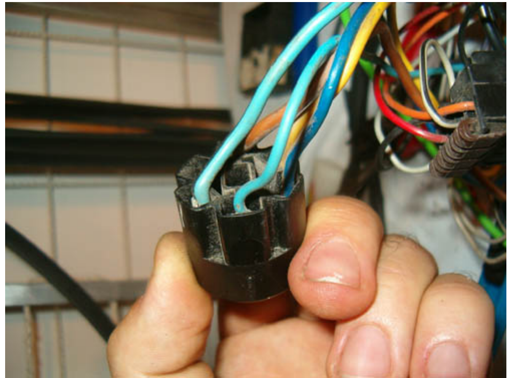
This is the heater fan switch connector. Strange enough there was no fault here.
